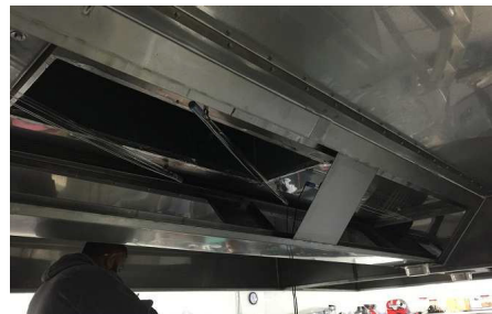
Inner view of the kitchen hood with UV system
