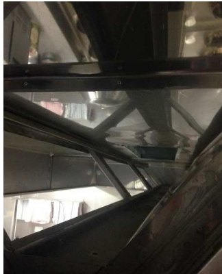
Inner view of the kitchen hood without UV system
